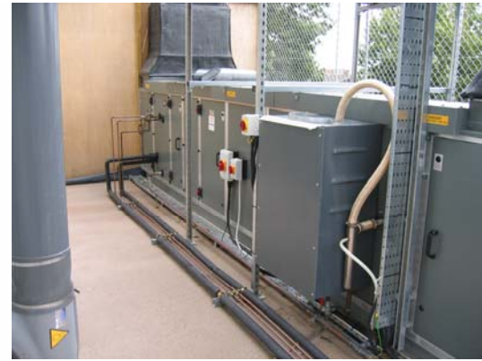
Air handling and conditioning plant can either be within a integral plant room or positioned externally to the building.
